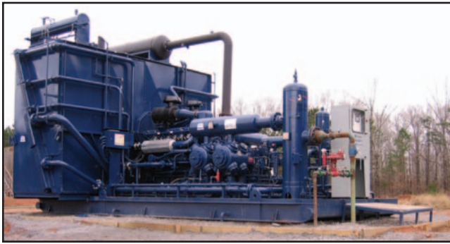
More recently, GE has begun installing its Jenbacher engines in mechanical drive applications. The first one, pictured here, is a J312 GMD gas engine driving a GE Oil & Gas Compressor.
