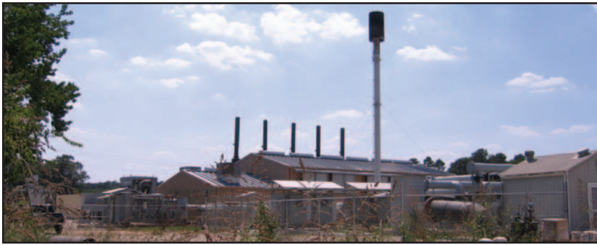
GE's Jenbacher gas engines are at home in electric power generation applications. Pictured is the Texas landfill project by Reliant Energy located near Humble, Texas, U.S.A. The site is comprised of five JGS 616 GS-L.L gas engines running on landfill gas with an electrical output of 1677 kW with an electrical efficiency of 38.3%.
